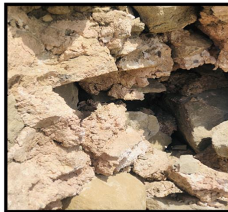
Figure 2 Deterioration of stone masonry of Ramkot Fort
